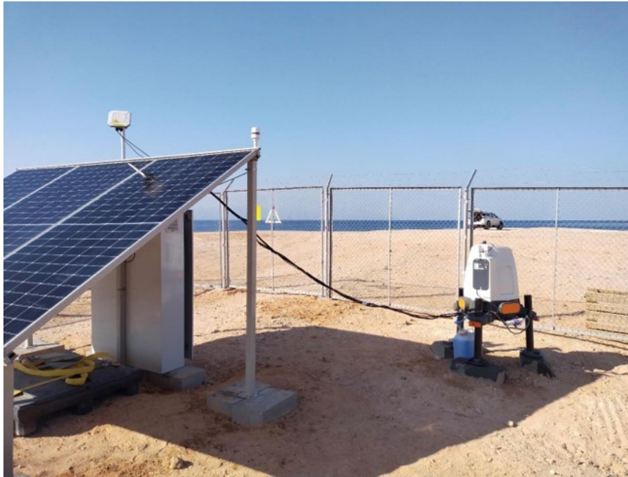
Figure 1: ZX 300 deployed with ENOWA in the Kingdom of Saudi Arabia
