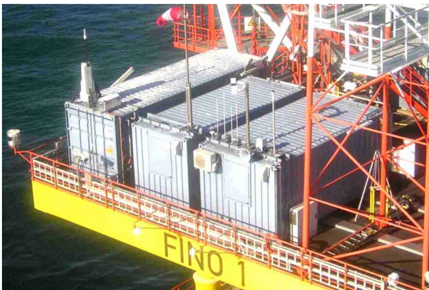
Figure 1: ZephIR on FINO-1 as mounted on the platform's Western most corner.
